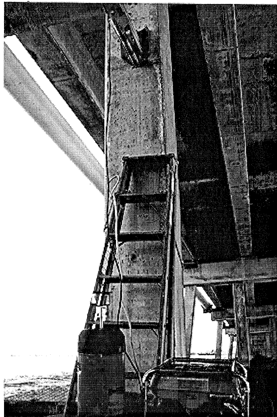
Figure I.7. Coring equipment set up at 10 ft. above high tide on a prestressed pile of the south bound Boca Chica Bridge located at the Florida Keys.
