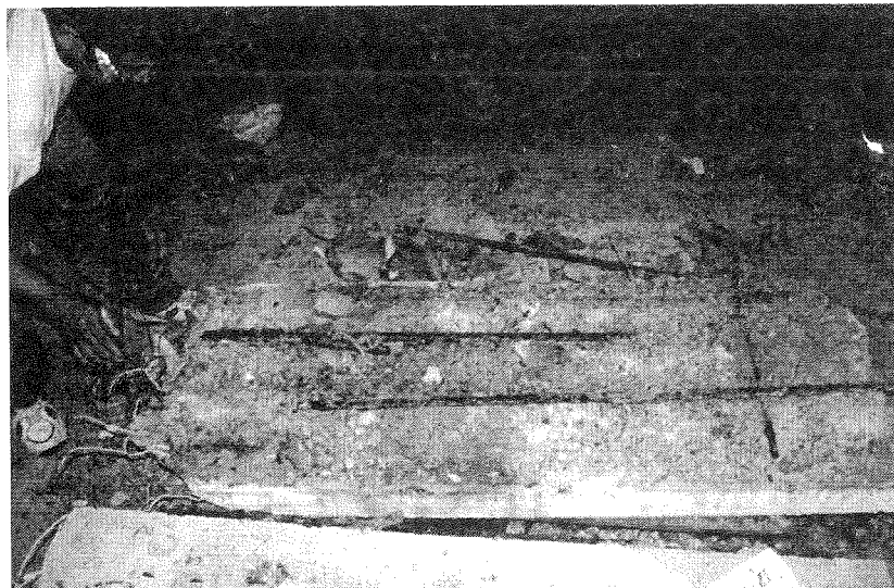
Figure 5 - Top mat of steel removed from all slabs for analysis.
