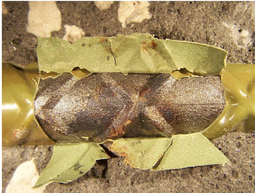
Figure 6. Typical steel and undercoating condition in disbonded ECR extracted from Sunshine Skyway Bridge, showing minor rust at coating breaks, and nearby discoloration of the metal surface. Trestle cap beam, 7.5 m AHT (SSK140E2).
