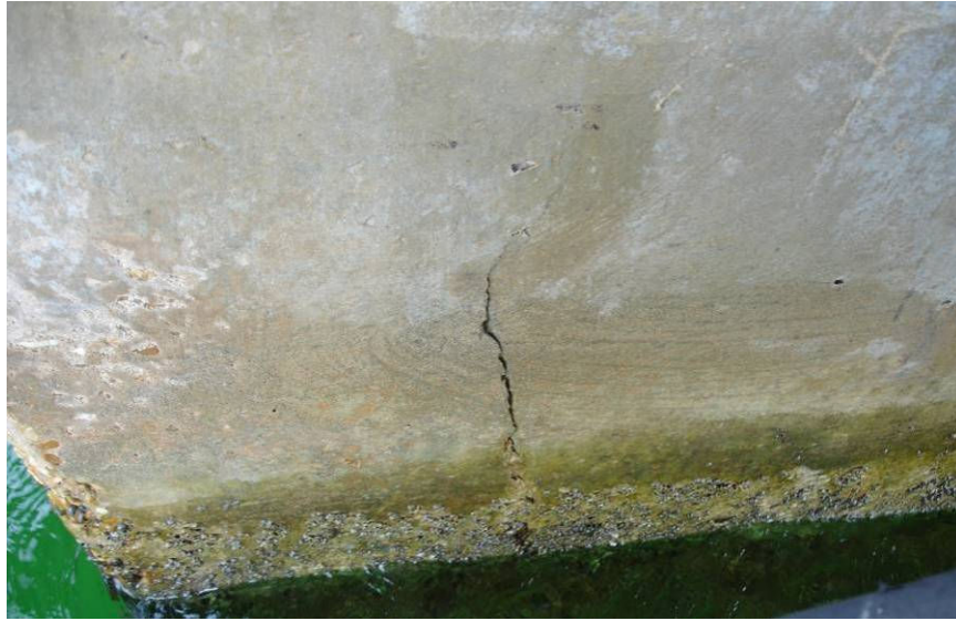
Figure 2. Large crack, >40 mils (1 mm) (Bridge over East Pass-Choctawatchee Bay).
