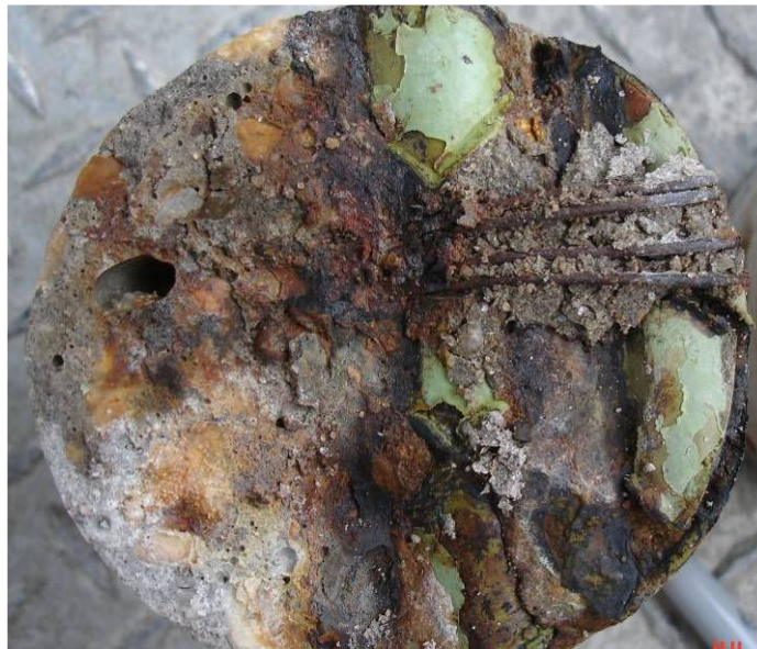
Figure 3. Extensive reinforcement corrosion. (Bridge over East Pass-Choctawatchee Bay Pier 29, North footer).
