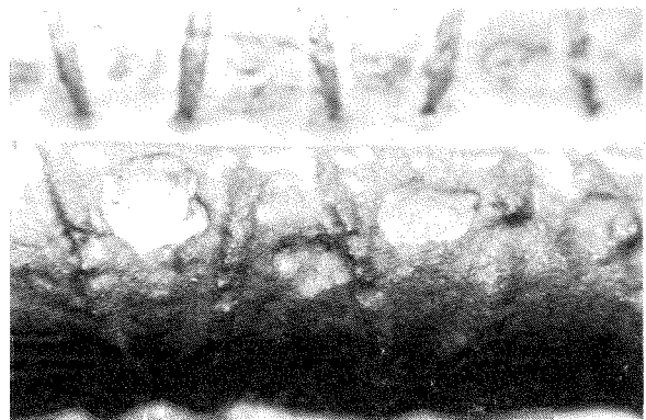
FIGURE 2 - Appearance of a #5 reinforcing bar (horizontal hoop portion of a bridge substructure column) after sandblasting.
