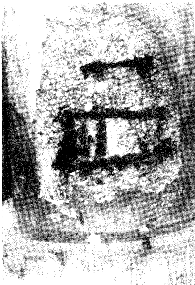
FIGURE 1 - General appearance of corrosion in a bridge column using epoxy-coated reinforcing steel.
