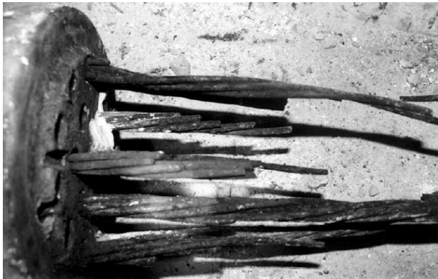
Figure 3 – Failed tendon-Niles Channel Bridge (June, 1999).
