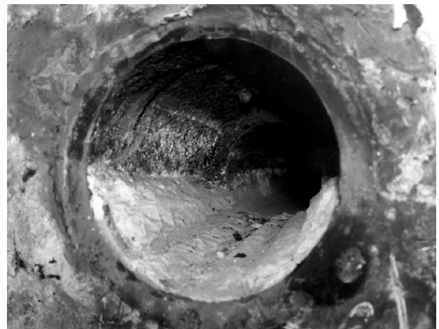
Figure 4 – Anchor at failed tendon showing chalky grout, partial grout filling and heavy corrosion.
