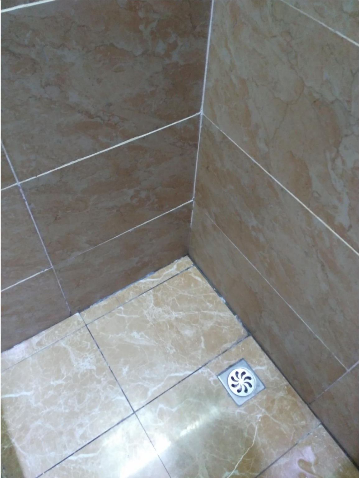
Figure 2. Typical Chinese shower floor with a drain, which doesn't have a trap.
