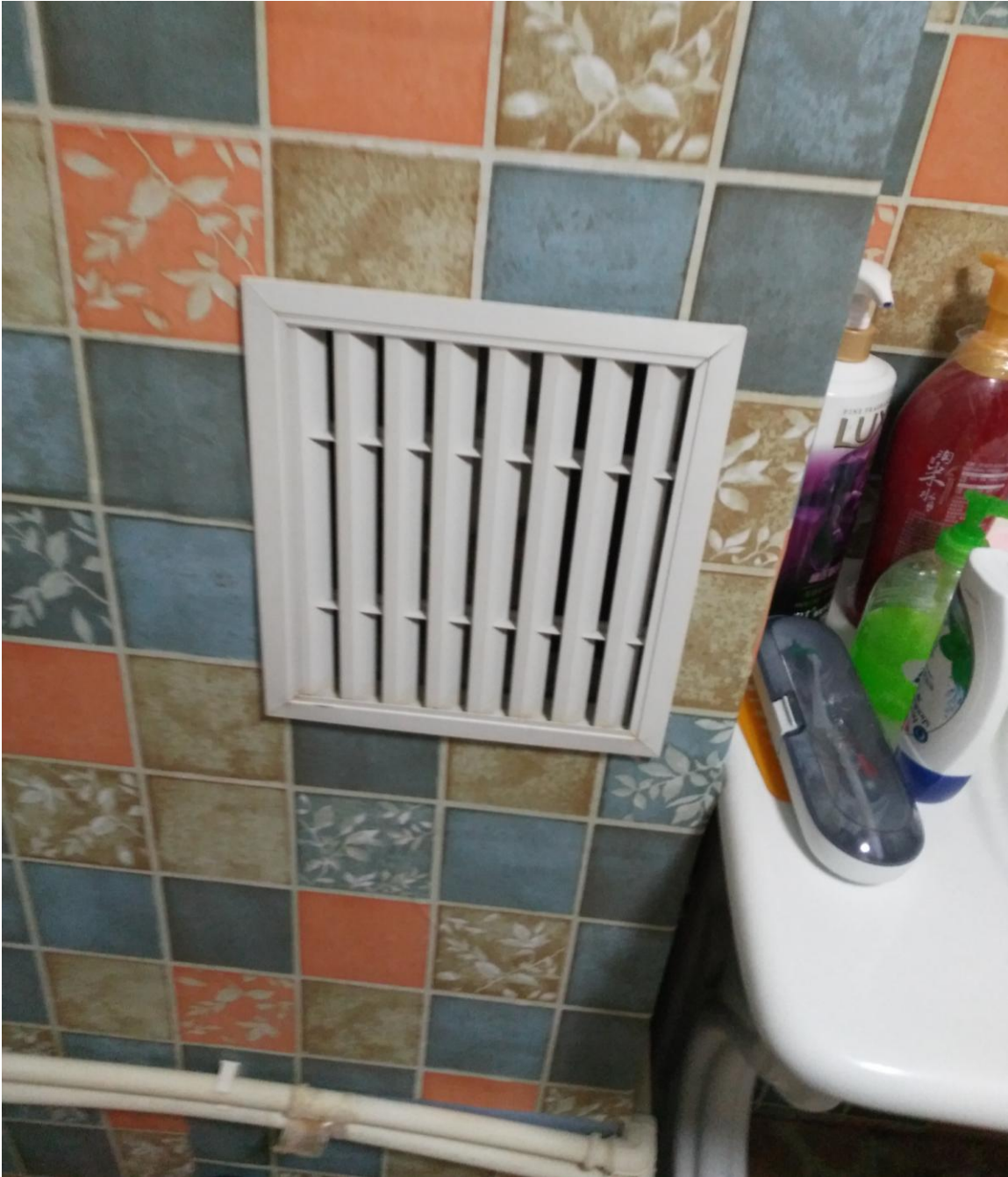
Figure 4. Bathroom vent carrying offensive odors from other apartments.
