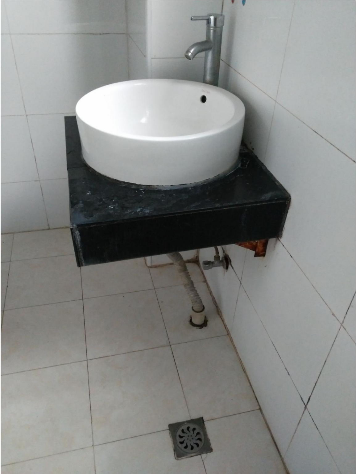
Figure 1. Photo of a typical Chinese bathroom showing a sink without water trap, unsealed sewage line and floor drain without a trap.
