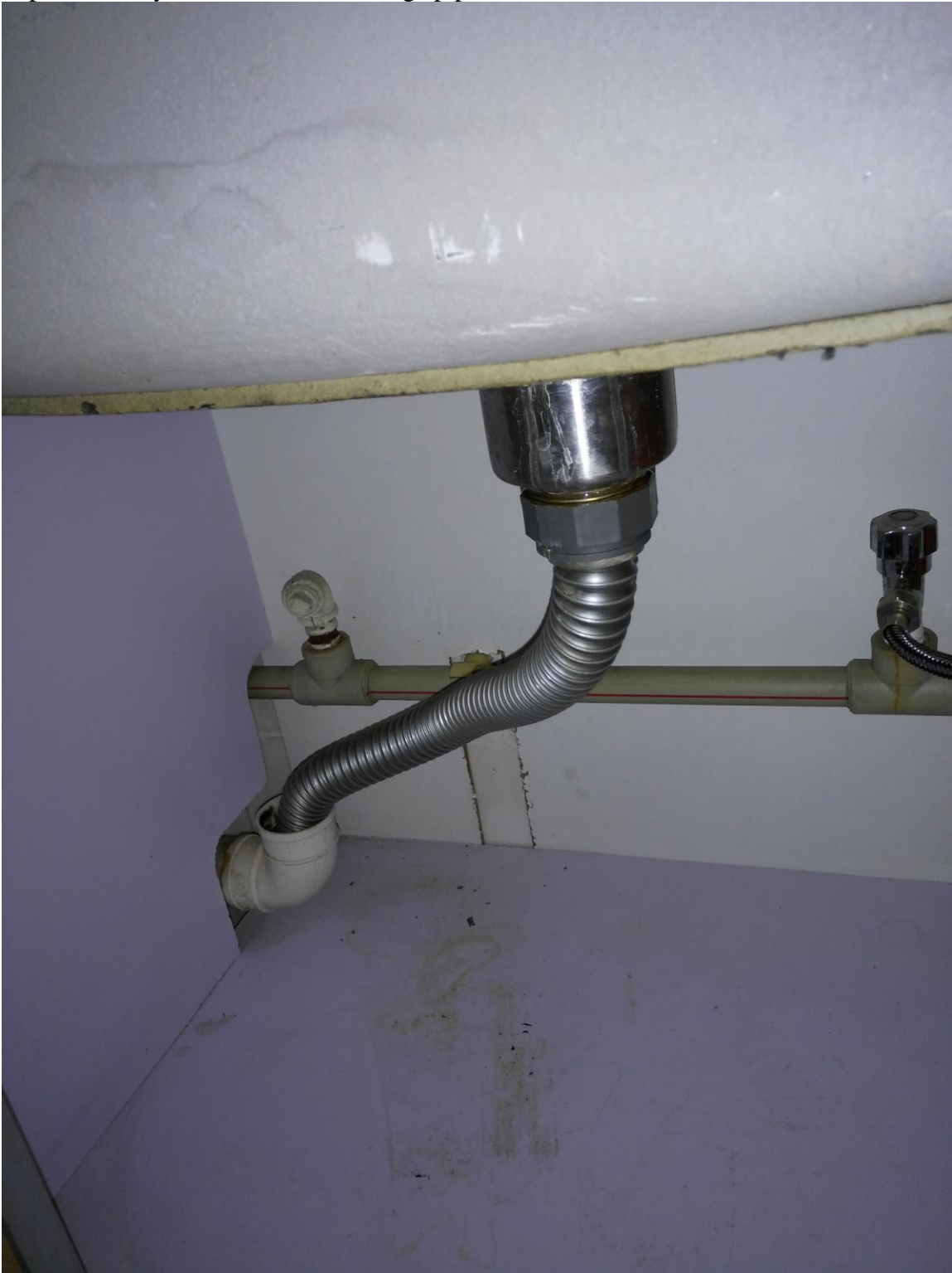
Figure 3. Flexible pipe connection in the kitchen without the water trap showing exposed unsealed drain pipe.
